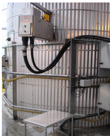
Figure 1: View of Model 83i probe at southeastern cement kiln
